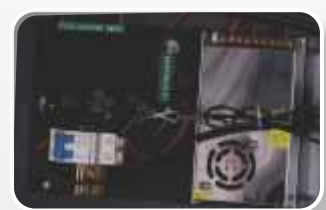
Pre Programmed Control Unit
